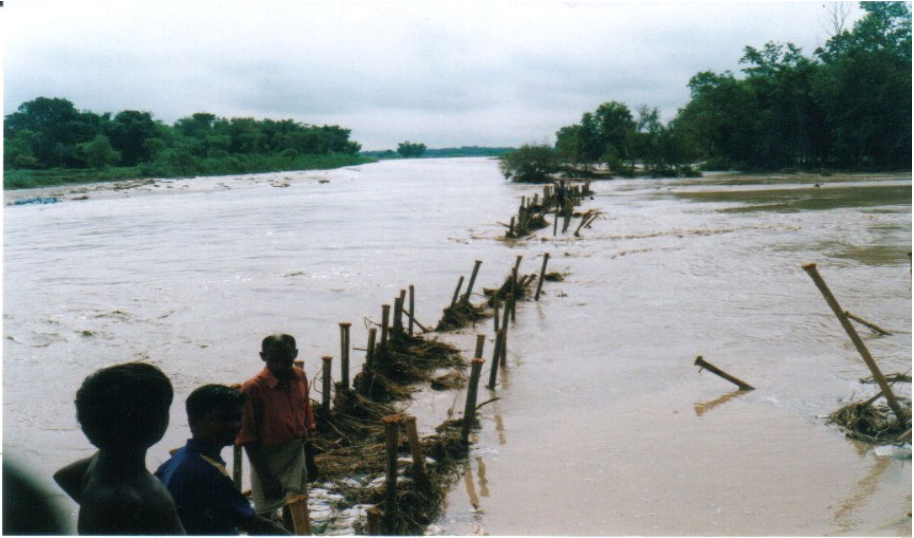
The above embankment in the flood the next day
