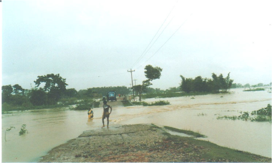
The main road to India from the village under flood
